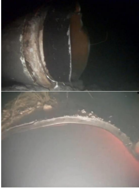
Figure 6. Destruction of the Nord Stream-1 pipeline section, initial inspection results Source: Nord Stream AG
